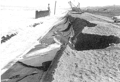
Photo 1 Seawall failure on Oarai Coast
